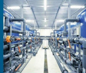
SEWAGE & WATER TREATMENT
